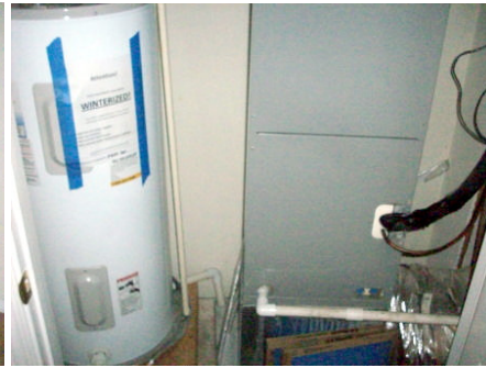
Boiler and Air Con System
